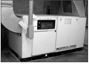
Ingersoll Rand SSR-EP100 100HP Air Compressor
